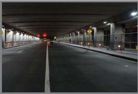
After: T.F. Green Airport, Warwick, R.I., upgraded its roadway lighting, reducing energy consumption by more than 50 percent.
